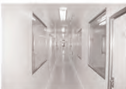
Class 100 Clean Room
